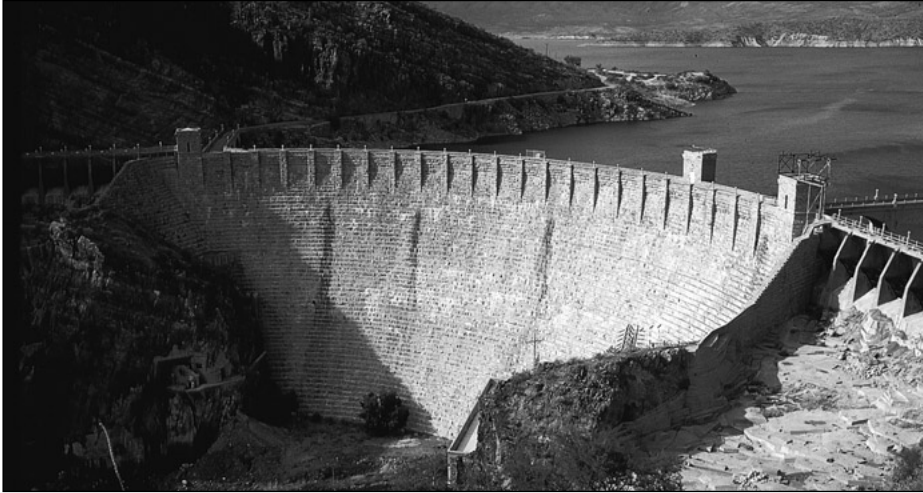
Roosevelt Dam in Arizona. Hydrostatic pressure, due to the weight of a standing fluid, can cause enormous forces and moments on large-scale structures such as a dam. Hydrostatic fluid analysis is the subject of the present chapter. ( Courtesy of Dr. E.R. Degginger/Color-Pic Inc. )
