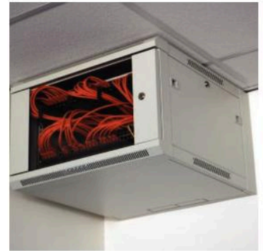
Figure 3.3.2 Network equipment is stored in special cabinets
