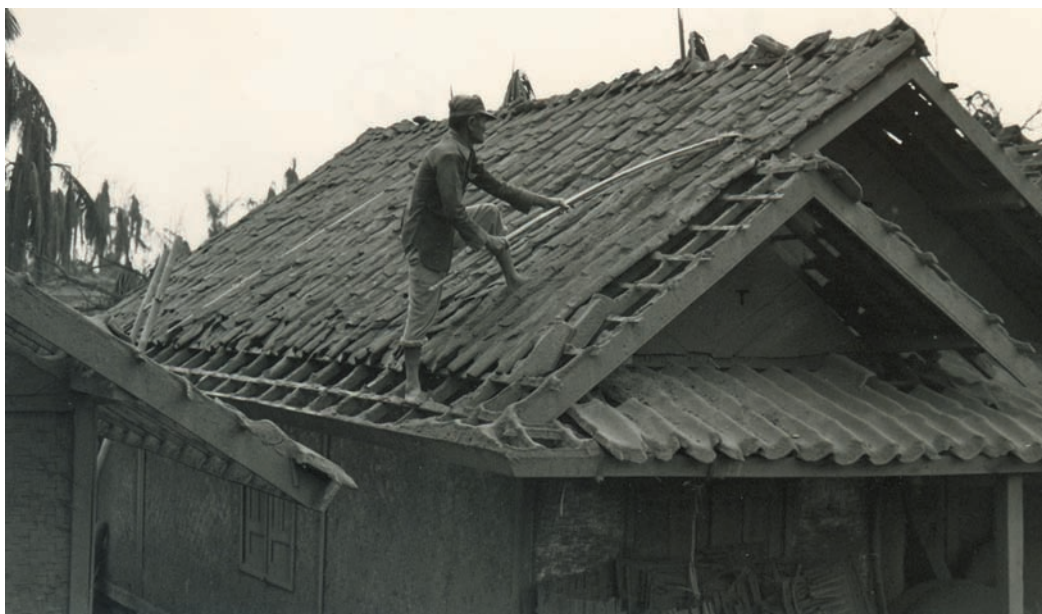
Fig. 14.15 Villager removing accumulated ash from his roof in Cikasasah between eruptive episodes of Galunggung volcano in 1982. People who returned to their homes after eruptive episodes to remove ash generally were able to save their homes from destruction. USGS photo by J. P. Lockwood.
