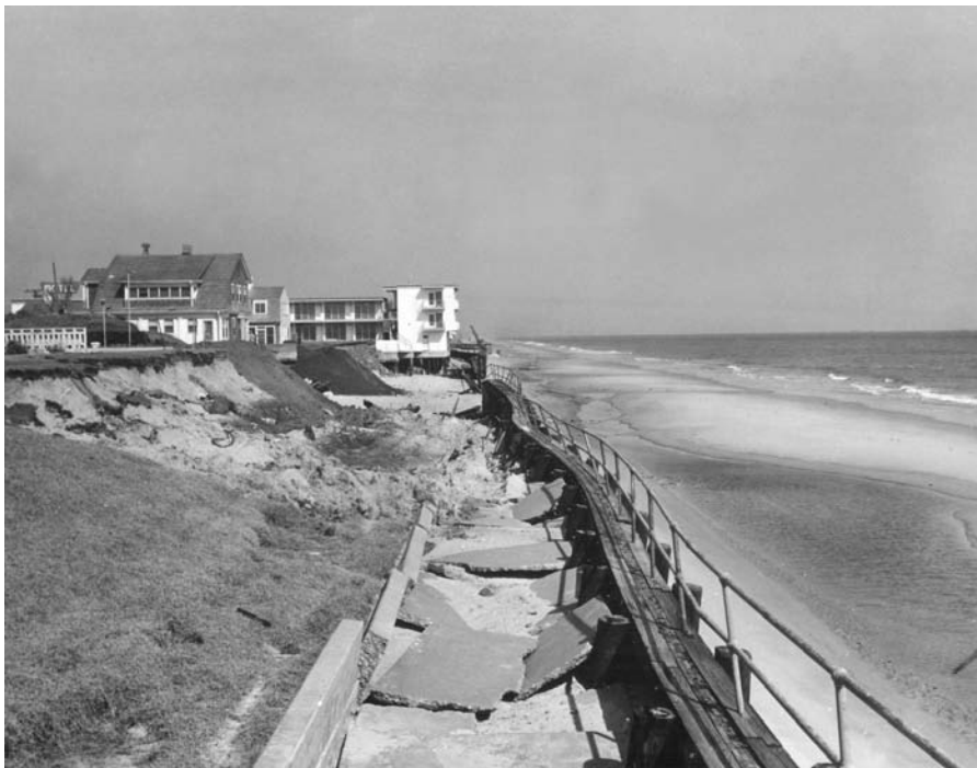
Figure 128 Damage to a beach area by storms and high tides at Virginia Beach, Virginia.
