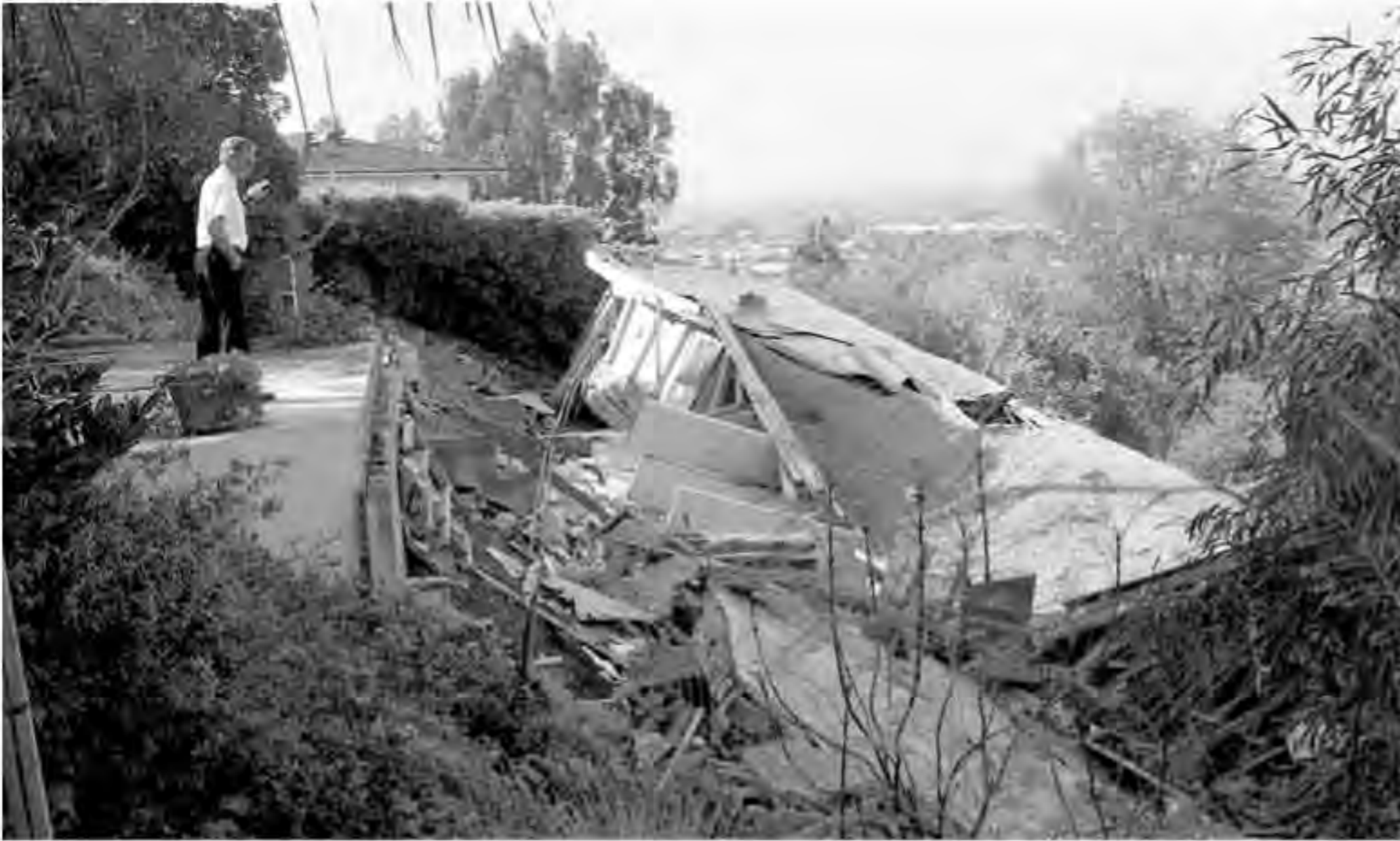
Los Angeles City Fire Department chief looks over the remains of an unoccupied house. The house, partially knocked off its foundation in the January 17, 1994, Northridge earthquake, fell completely off its foundation in the strong aftershock, which registered 5.3 on the Richter Scale. AP/Wide World Photos.
