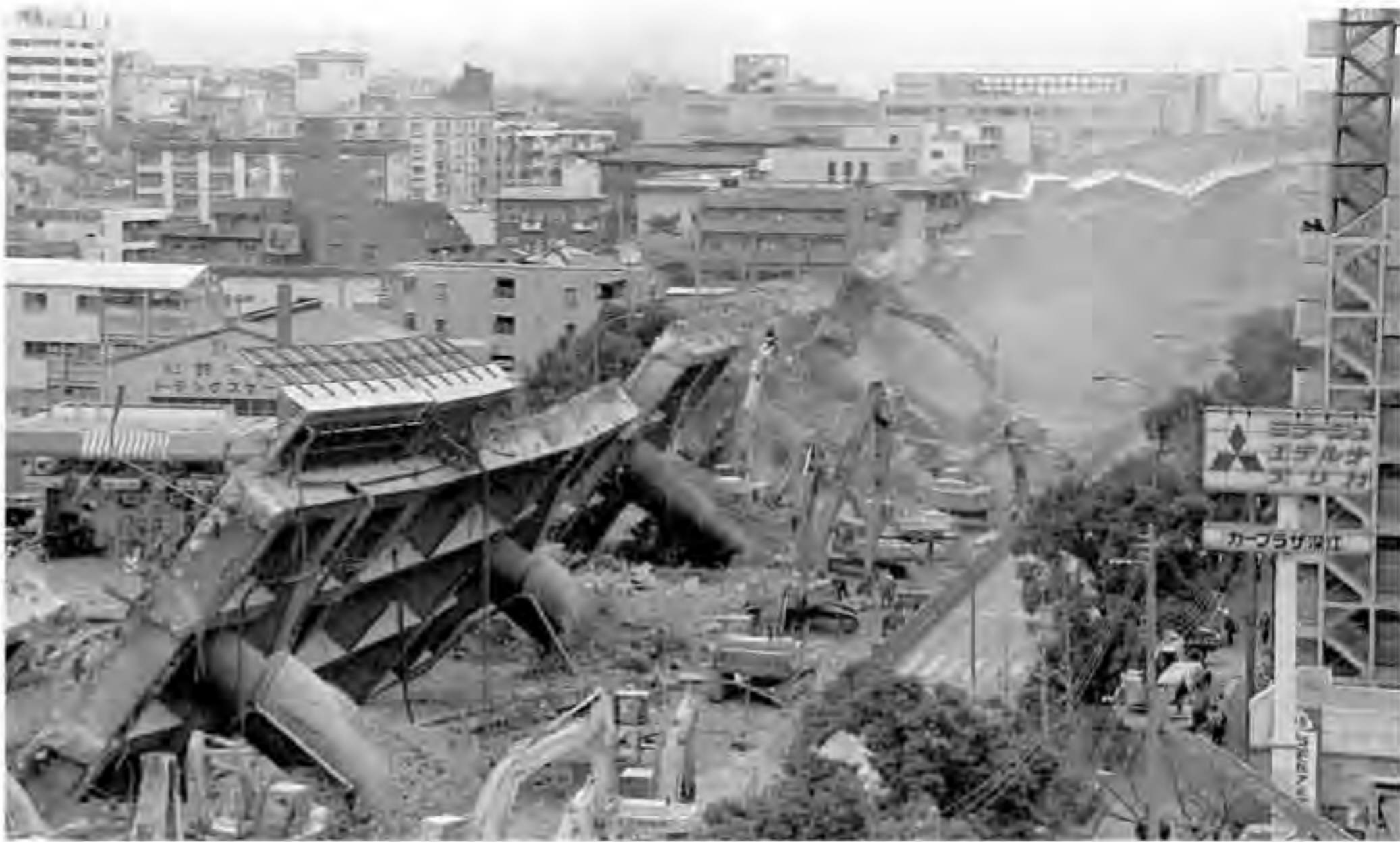
Heavy construction machines break up concrete from a toppled freeway in Kobe, Japan. Portions of the Kobe-Osaka freeway collapsed during the earthquake that hit this western Japanese city early on January 17, 1995. AP/Wide World Photos.
