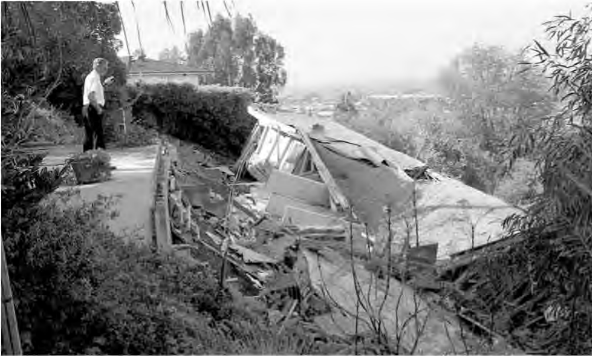
Los Angeles City Fire Department chief looks over the remains of an unoccupied house. The house, partially knocked off its foundation in the January 17, 1994, Northridge earthquake, fell completely off its foundation in the strong aftershock, which registered 5.3 on the Richter Scale. AP/Wide World Photos.
