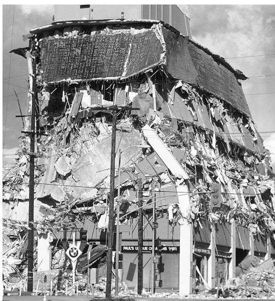
This building was severely damaged in the 1994 Northridge, California earthquake. (Joe Sohm Visions of America/Newscom)
