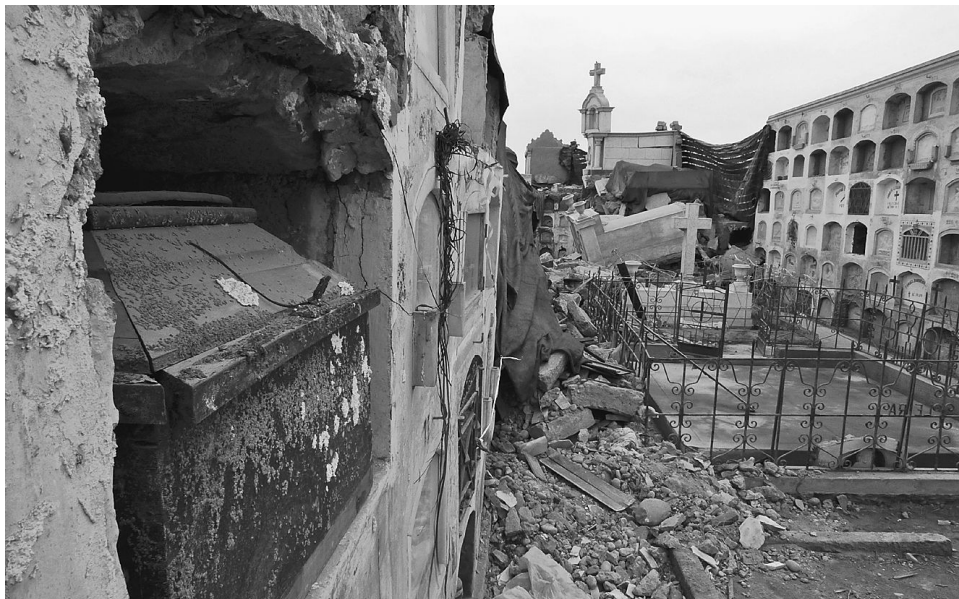
Graves at the General Cemetery of Pisco, Peru, damaged in a 2007 earthquake in the region. (Ric Francis/ZUMA Press/Newscom)
