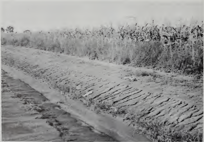
FIG. 22.18. Photo of a road cut in which the much greater erisibility of the plastic B horizon in a soil profile is shown by the change from sheet erosion to gullyng. (Photo by Engineering Experiment Station, Purdue University.)
