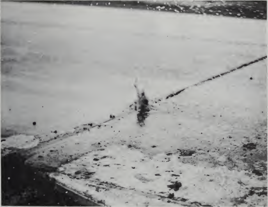
FIG. 22.10. Ejection of a mud-water mixture (pumping) from a concrete pavement joint immediately after passage of a car. (Photo by Engineering Experiment Station, Purdue University.)
