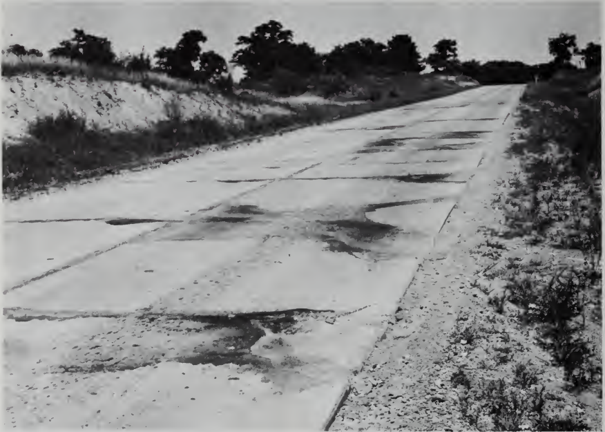
FIG. 22.11. Deterioration of a highway built upon a clay-shale subgrade. (Photo by Engineering Experiment Station, Purdue University.)
