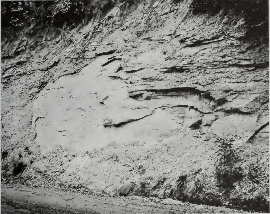
FIG. 3.2. Exfoliation of massive siltstone. Alternate freezing and thawing are mainly responsible for the spalling off of the rock surface. (Photo by P. B. Stockdale.)
