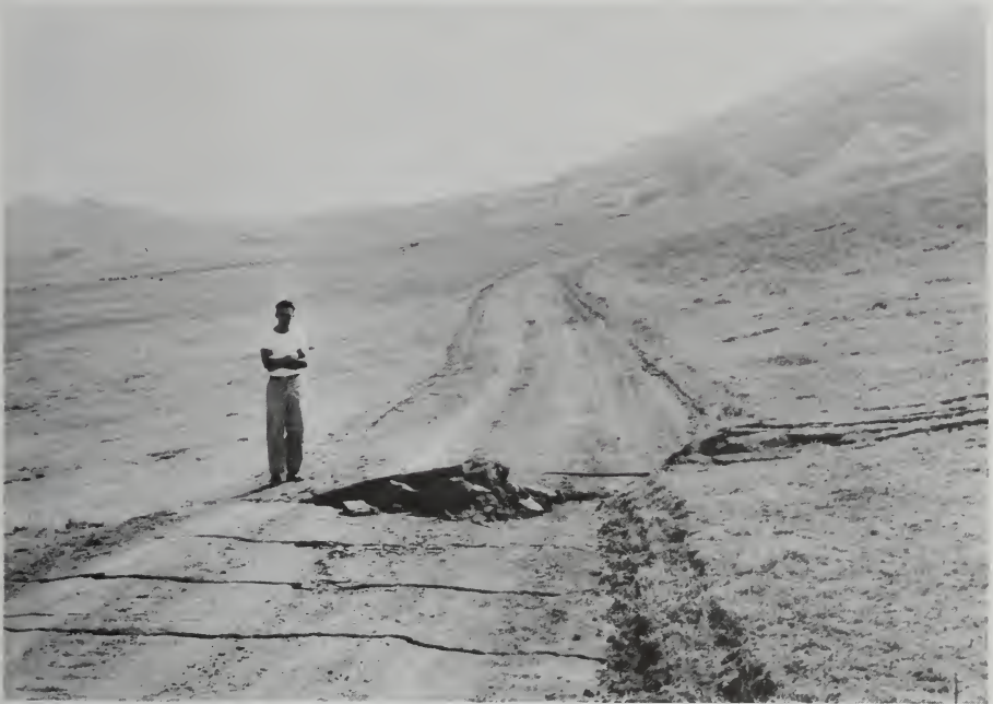
FIG. 10.12. Lateral displacement of road near Arvin, California, caused by the Arvin-Tehachapi earthquake of July 25, 1952. (Photo by R. C. Frampton.)
