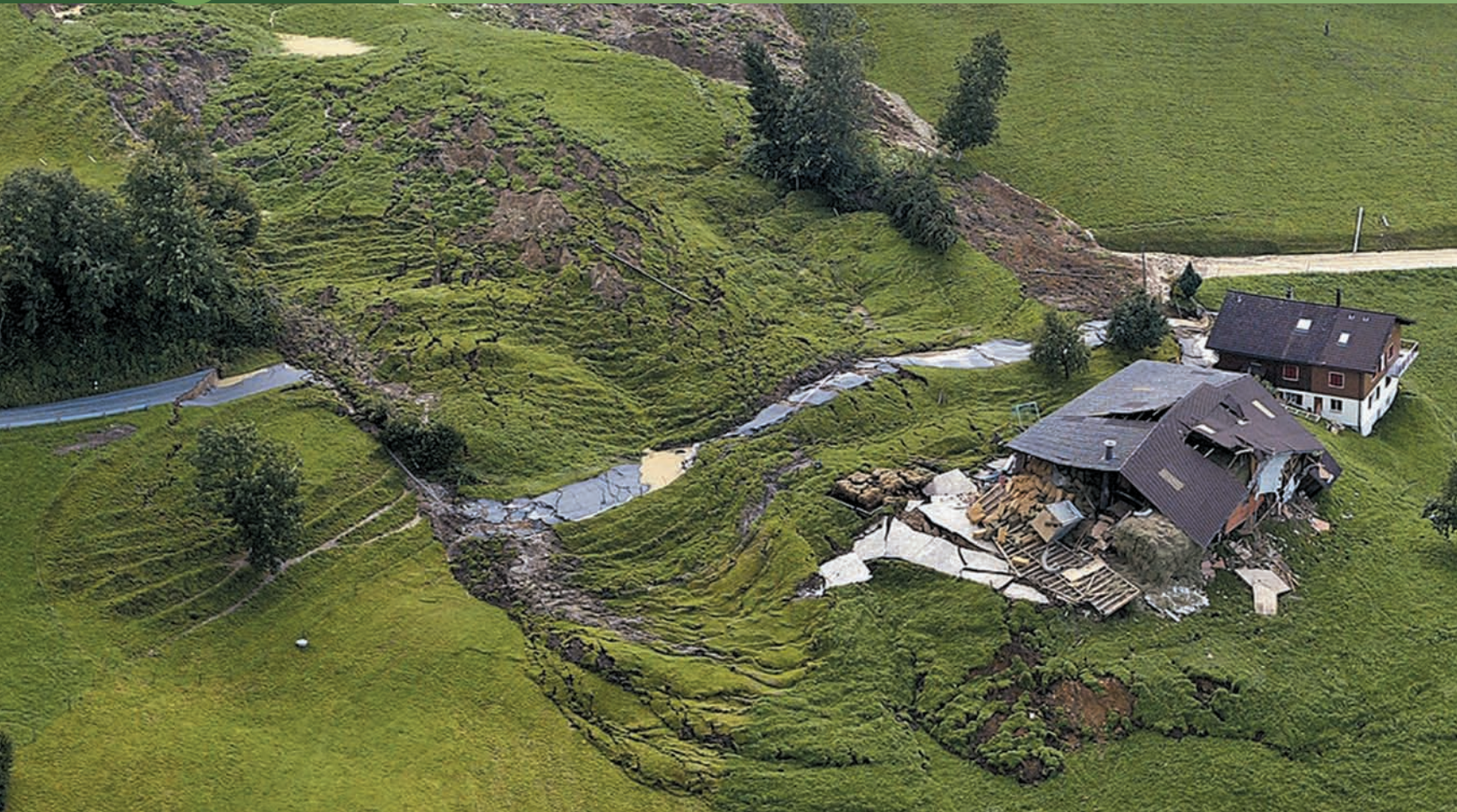
A farm house and stable are damaged by a landslide outside the town of Entlebuch, central Switzerland, Tuesday, Aug. 23, 2005. Note the displaced segment of the road. This landslide is an example of a slump-earthflow described in this chapter. Photo © AP/Wide World Photos
