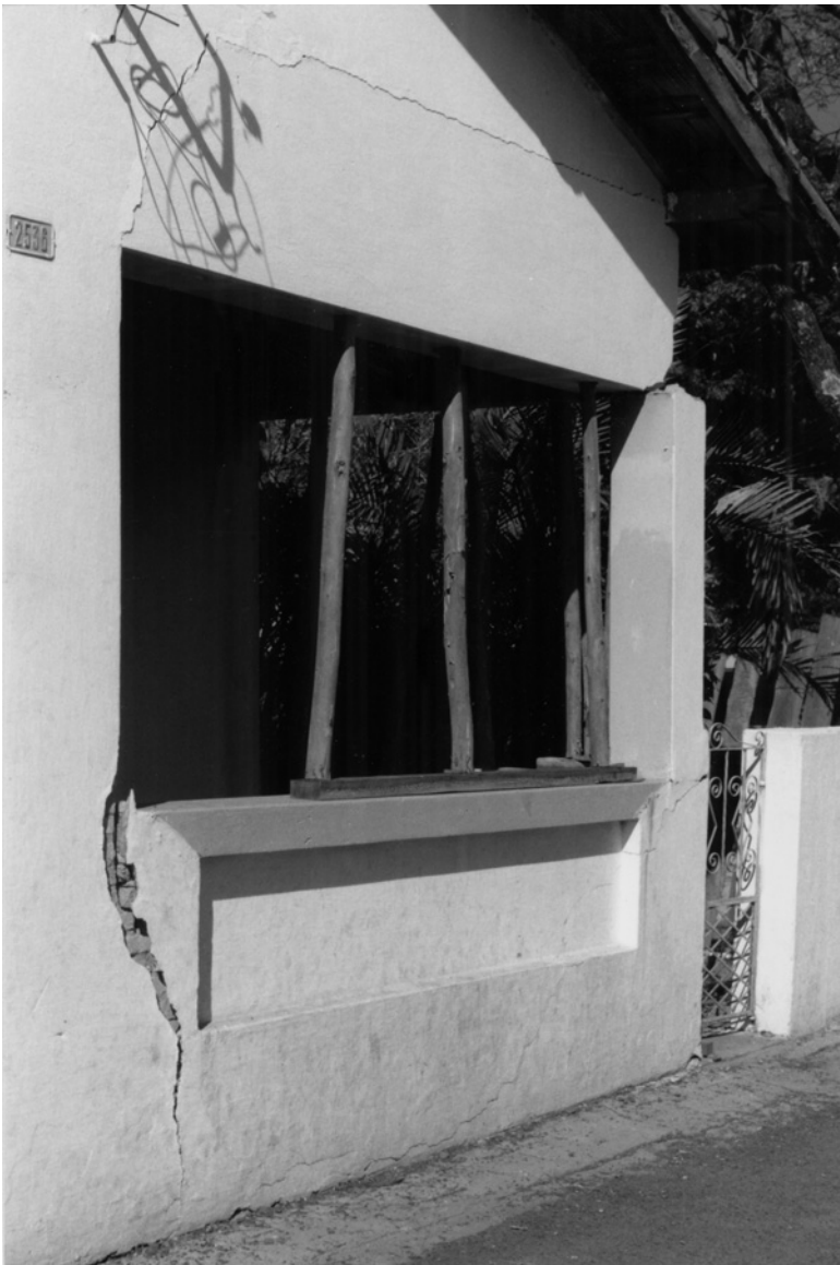
Fig. 9.18. Settling of a house wall on collapsible, tropical oxisoil in Rio Claro, Sao Paulo, Brazil. Note cracks in wall and wooden supports in windows
