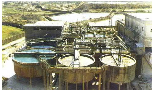
FIGURE 14.15 Effluent treatment plants to recover metals and recycling of water for industrial uses, Rajasthan, India.
