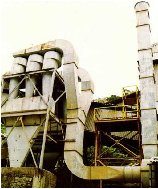
FIGURE 14.8 Air pollution control by a dust extraction system installed at an ore-dressing plant, India.
