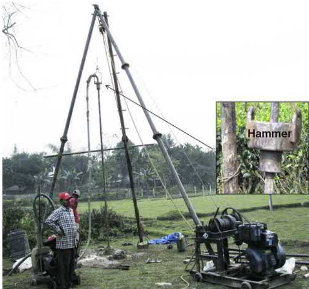
FIGURE 7.2 Percussion drilling in operation for rock quality and quick target test for mineral occurrences at low cost and reduced time. The hammer is detailed in the inset.
