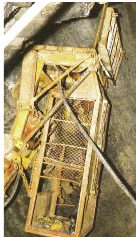
FIGURE 12.12 Alimak raise climbers are often in use for vertical or inclined excavation to join between levels and sublevels.
