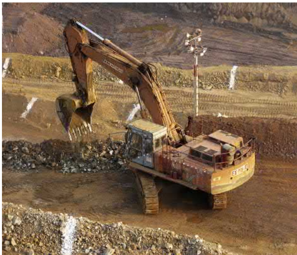
FIGURE 12.39 Hydraulic crawler-mounted medium-sized mucking and loading unit in operation at Sukinda chromite mine bench.
