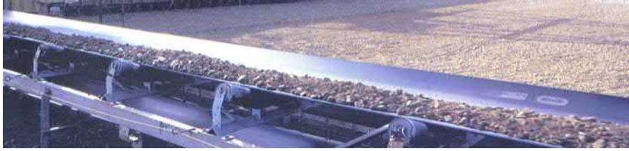
FIGURE 13.1 Standard open surface rubber belt conveyor system with support rollers at the bottom of the belt for ore transportation over kilometers.
