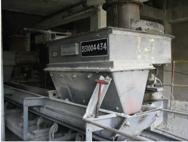
FIGURE 13.16 Close circuit transfer of oversize material from secondary crusher collected in an ore bin (top) and autotransfer to tertiary crusher by a conveyor belt (bottom).
