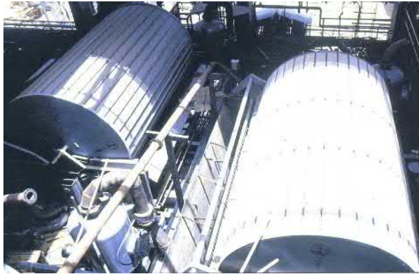
FIGURE 13.50 A view of a drum filter, an alternative process of dewatering concentrate.
