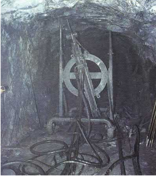
FIGURE 12.30 Column-mounted pneumatic screw feed Simba Junior drills suitable for underground mines to drill in 360-degree rotation at Rajpura-Dariba mine, India.
