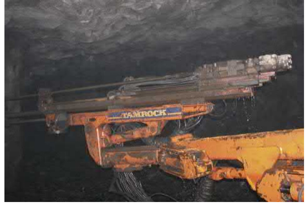
FIGURE 12.32 Close view of single hand-operated face drilling by Tamrock single boom electric-powered jumbo drill with straight 14 feet steel feed operation at Sindesar-Khurd mine, Rajasthan, India.
