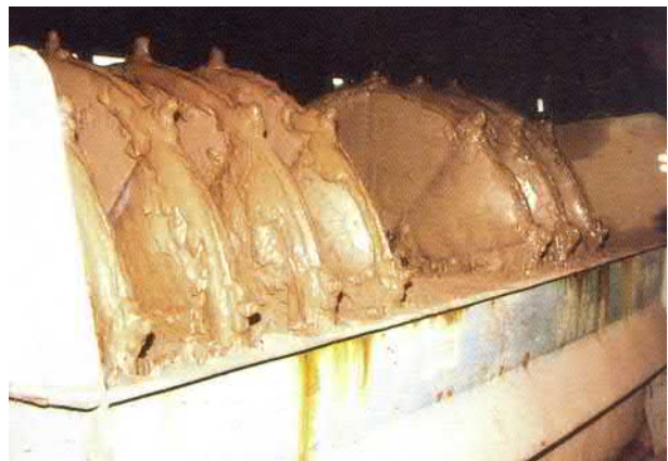
FIGURE 13.49 A view of a disc filter in the second phase of dewatering of concentrate.
