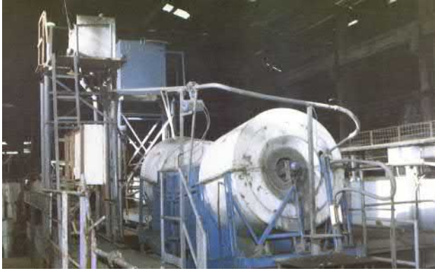
FIGURE 13.33 Multigravity separators at Rajpura-Dariba mineral process plant in India during the early 1990s.
