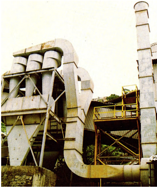
FIGURE 14.6 Air pollution control by dust extraction system installed at ore dressing plant, India.
