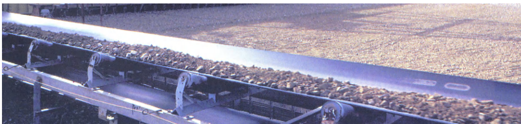
FIGURE 12.1 Standard open surface rubber belt conveyor system with support rollers at the bottom of belt for ore transportation over kilometers.
