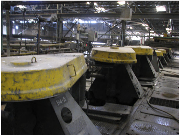
FIGURE 12.40 A typical bank of flotation cells in operating circuit.
