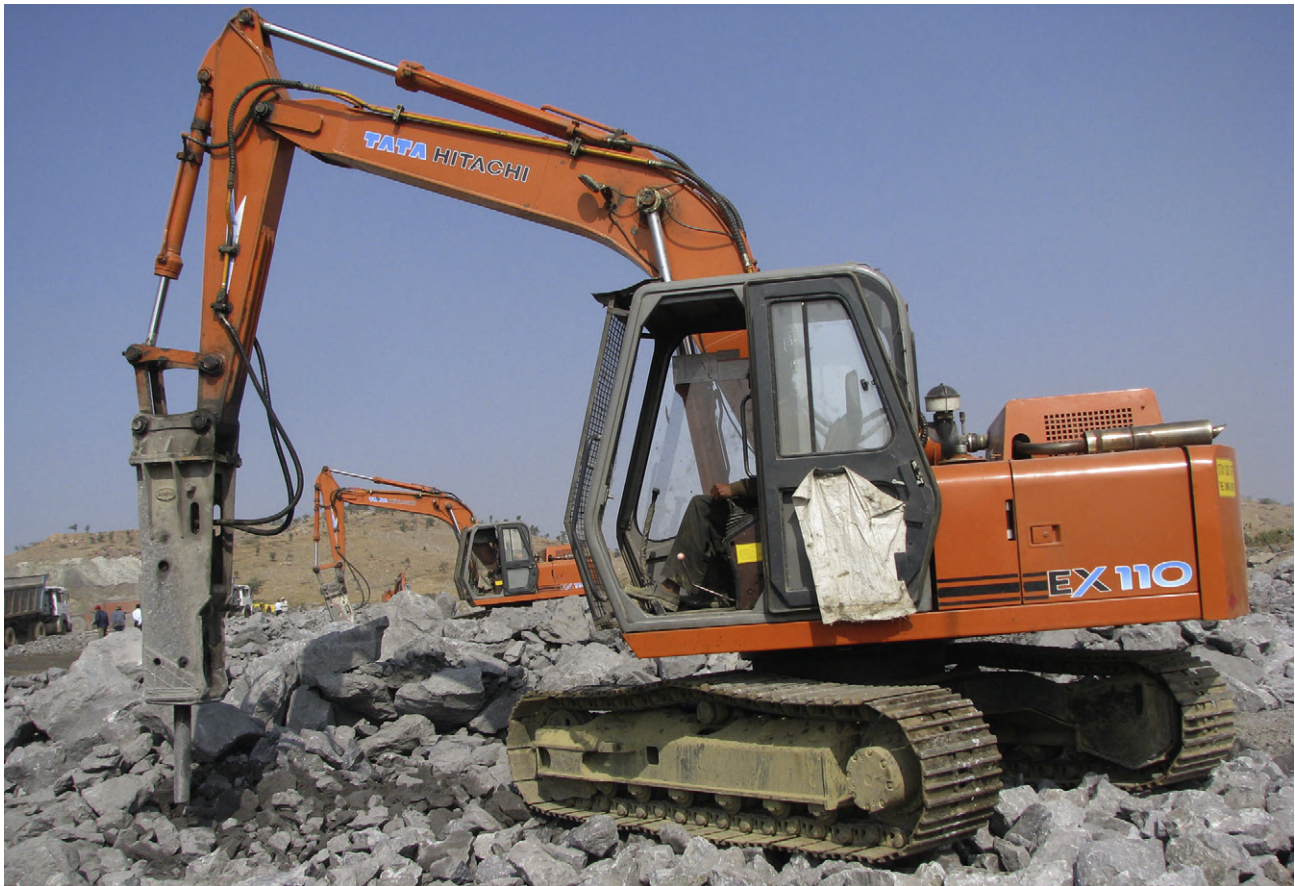
FIGURE 11.34 Crawler-mounted (continuous tracks) hydraulic hammer type Rock breaker in operation to break large size stones of ROM ore at mine outside.
