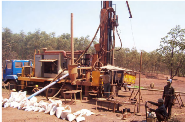
FIGURE 7.13 RC drilling in operation and sample collection for iron ore deposits (Credit: Biplab Mukherjee).
