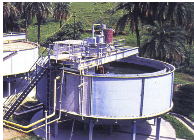
FIGURE 12.50 A view of thickener with rake mechanism in the first phase of dewatering of concentrate by sedimentation or gravity settling of solids.
