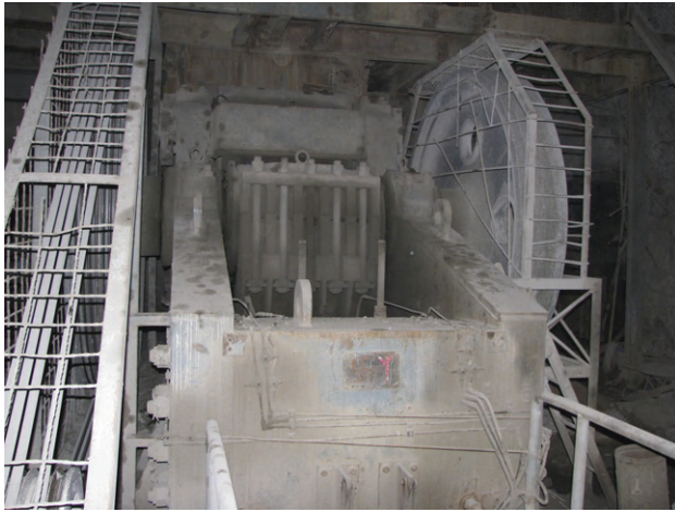
FIGURE 12.10 Medium size Jaw crusher in operation in underground mine for crushing ROM ore before transferring to surface at Zawarmala, India.
