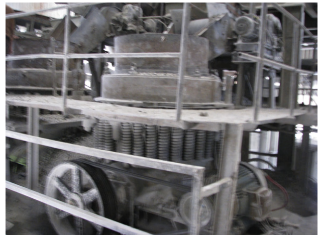
FIGURE 12.13 A working Cone crusher in operation and performing both secondary and tertiary crushing function.
