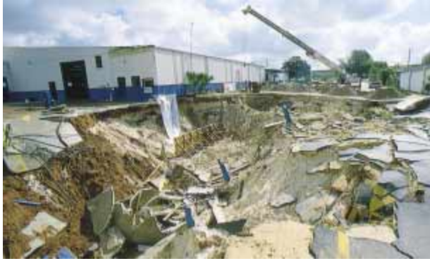
Figure 15-11 A dropping water table caused subsidence and structural damage in Jacksonville, Florida. (Wendell Metzen/Bruce Coleman, Inc.)
