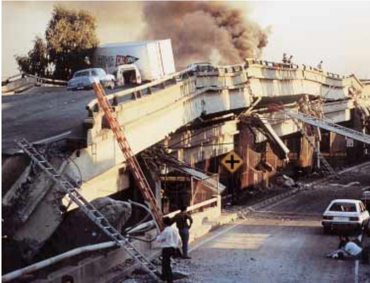
Figure 10-9 Surface waves cause a large proportion of earthquake damage. Collapse of Interstate Highway 880 during the 1989 Loma Prieta, California, earthquake. (Paul Scott/Sygma)
