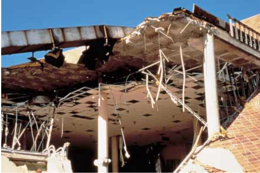
Figure 10–22 The January 1994 Northridge, California, earthquake killed 55 people and caused eight billion dollars in damage. (Earthquake Engineering Institute)
