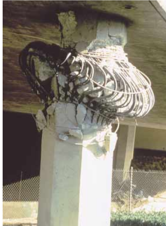
Figure 1–12 Earthquake-resistant design allowed this bridge support to rupture during the 1994 Northridge, California, earthquake, but prevented total collapse of the bridge. (Earthquake Engineering Research Institute)
