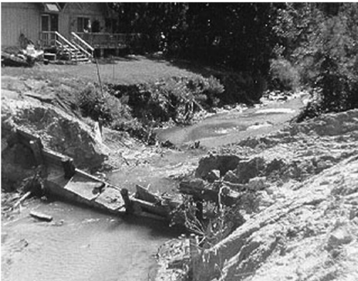
Fig. 7. Collapsed check dam in Lake Forest Subdivision (Photo: J. Carlton, August 31, 1979).
