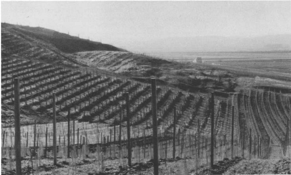
Fig.7.1. The landslide of Im Laberstall in the Tertiary basin of Mainz, dating from January 1989. Its volume is about 125\,000\text{m}^3 , the height of the scarp about 6-7m (R.Dikau, 1990).
