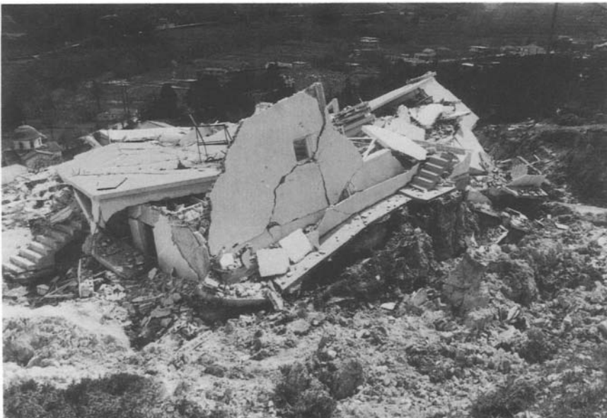
Fig.9.7.A ( upper ): Rotational slides in marly Neogene sediments, transformed into earthflows near the foot which abut on the Preveza-Igoumenitsa road, western Greece. B ( lower ): Collapsed house built on clayey-marly Neogene sediments
