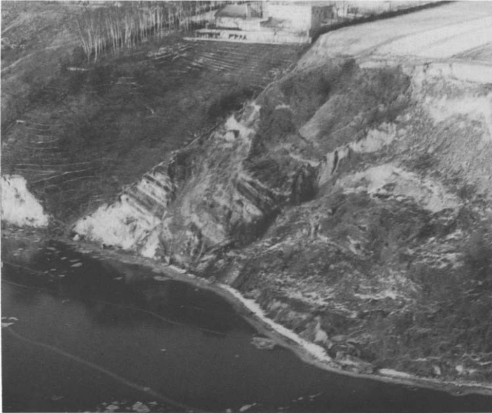
Fig.15.10. Mass movements on the bank of the Włocławek reservoir at Dobrzyn, triggered by the raised water level (photo M.Grześ)
