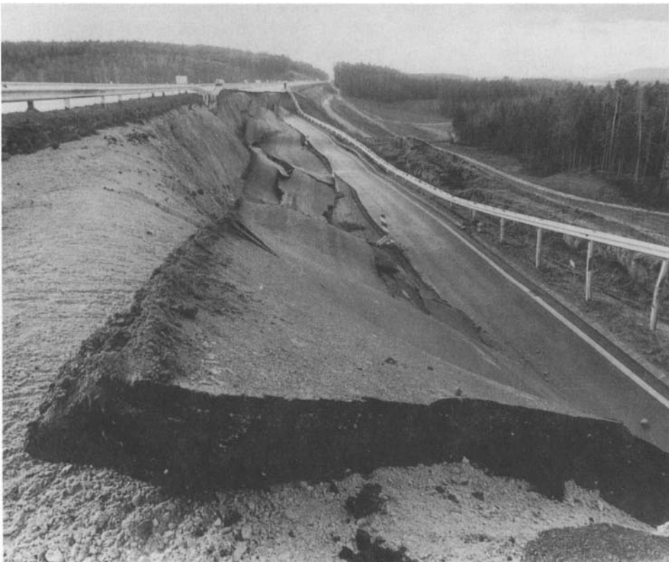
Fig.1.7. A section of the newly-built Süd-Autobahn which collapsed in December 1985, a few days after the road was opened (Copyright, Franz Pauritsch)
