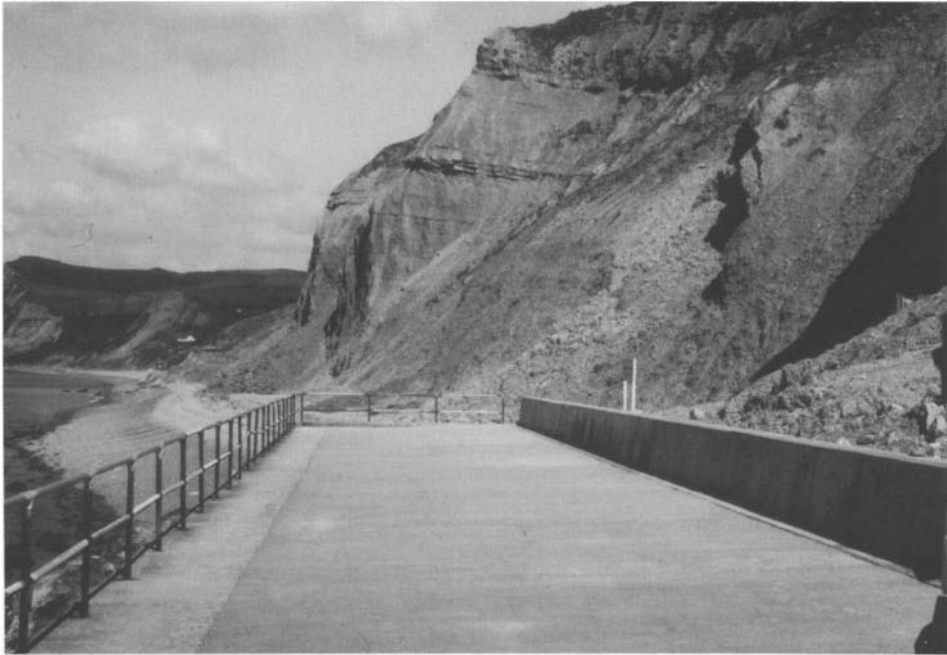
Fig.8.8. The western end of the sea wall at West Bay, Dorset, built to protect the cliffs (Jurassic) from wave attack. Large boulders (not visible) have been placed beyond the end of the wall, but the sea is already beginning to attack the exposed end and the sediments behind. The cliffs beyond are unprotected and may be expected to retreat, thus further increasing the vulnerability of the wall. (Photo: C.Embleton)
