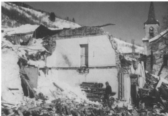
Fig.6.8. Buildings destroyed by snow avalanches, 20 January 1981, in Saint Colombanles-Villards, Savoy (photo: F.Valla)
