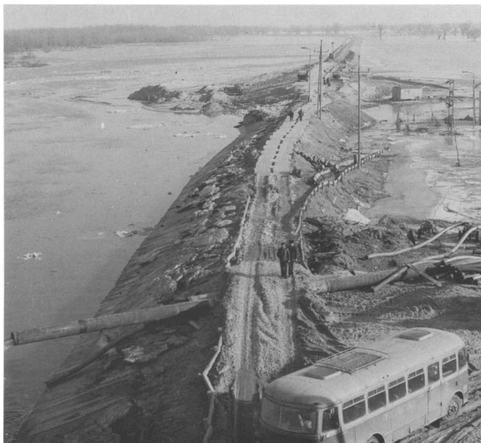
Fig.15.4. Destruction of Vistula dyke by the catastrophic ice-jam flood of January 1982. The photo was taken in March showing repairs under way (photo M.Grześ).
