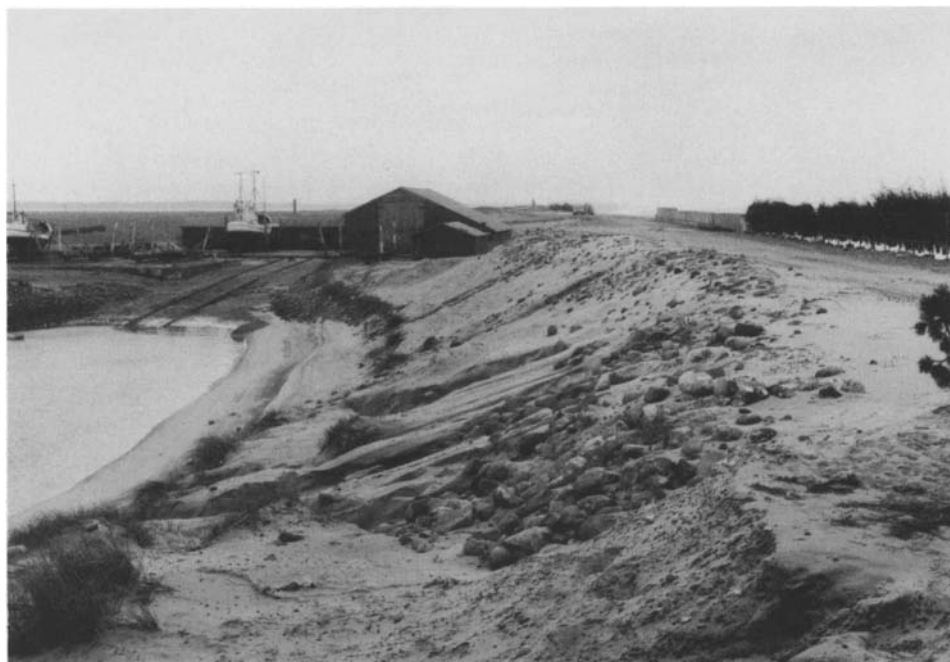
Fig.4.3. A dyke overtopped by waves, west of the fishing port of Torsminde (March 1990). The seaward side of the dyke is to the right (south); north of the small shipyard is a basin partly filled with sand transported across the dyke. Facing the North Sea, branches have been planted in a fence to prevent transport of blown sand, but most of the sand has been carried over the dyke by waves.
