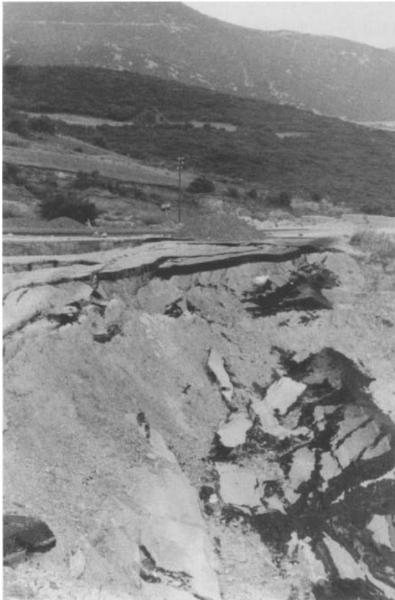
Fig.9.8. Failure of road embankment with poor foundations on weathered flysch and lacking drainage
