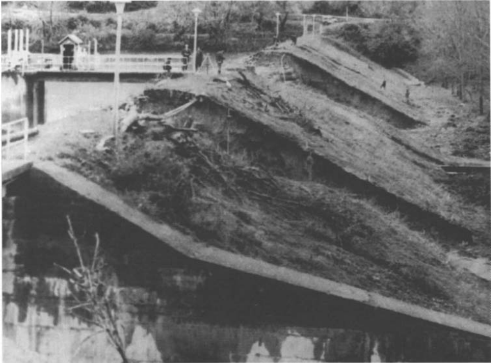
Fig.9.16. A view of the breaches in the Atras dam caused by the flood of 18-19 November 1979
