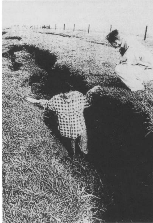
Fig.2.2. Damage to dykes along the Meuse caused by the Roermond earthquake of 13 April 1992 centred in the Campine area of the Netherlands
