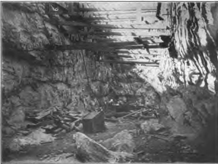
Fig. 28. Rapid Transit excavation, Broadway, 117th-118th Streets. Cut 25-30 feet deep in Manhattan gneiss. June, 1901.
