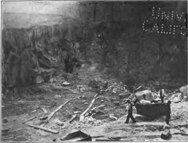
Fig. 2. Pennsylvania Railroad Excavation, 31st Street between Seventh and Eighth Avenues, looking South.
