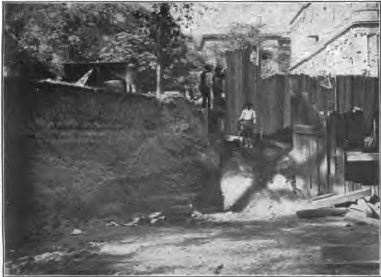
Fig. 55. Rapid Transit excavation in front of the City Hall, in sand, showing undisturbed bed of sand. June, 1901.
