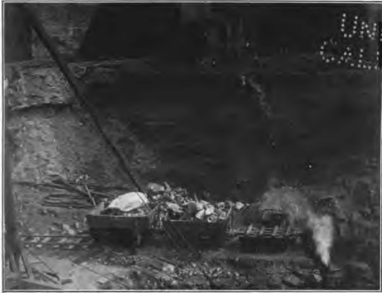
Fig. 54. Pennsylvania Railroad excavation, 33d Street east of Seventh Avenue. Cavities made by removed boulders in the sand bank. June, 1901.
