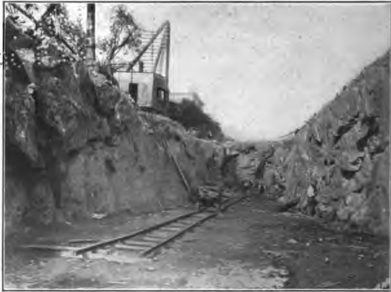
Fig. 29. Rapid Transit excavation at 145th Street, looking north to 147th Street. October, 1901.
