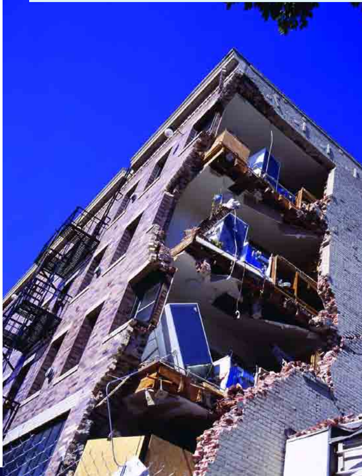
A damaged building after an earthquake.
