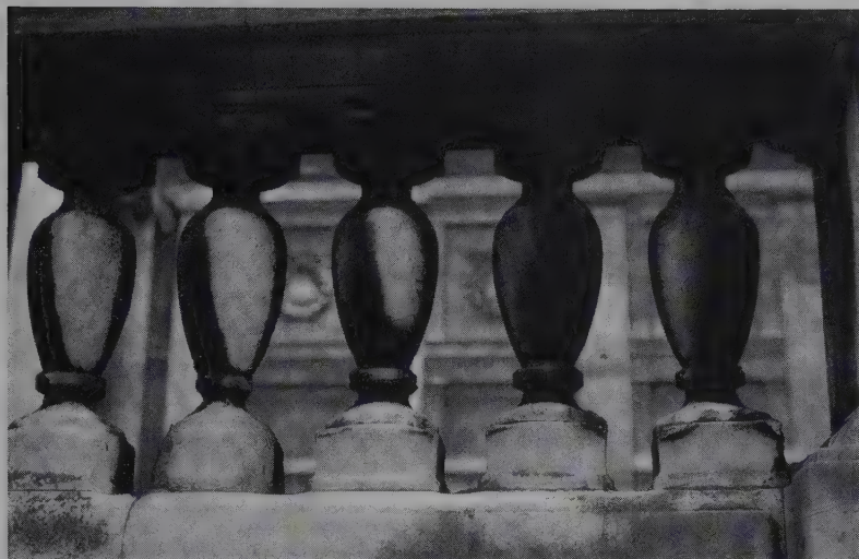
Plate 5.1 Weathered balustrade on the Ashmolean Museum, Oxford, England. The balustrade has now been cleaned.
