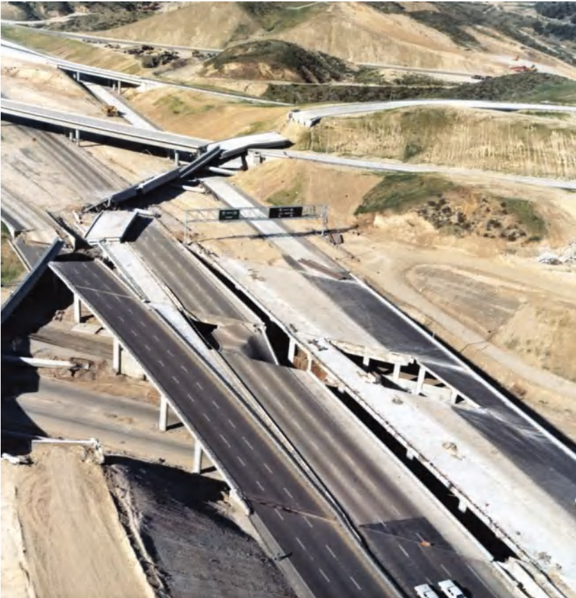
This California highway overpass collapsed during a 1971 earthquake. (R. Kachadoorian/USGS)
