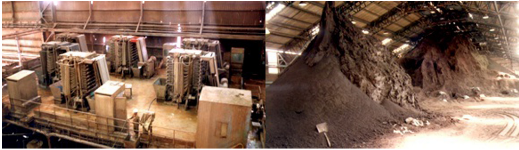
FIGURE A.17 Concentrate filters and the concentrate storage yard, Rampura-Agucha. Source: Photo courtesy by Gandhi.
