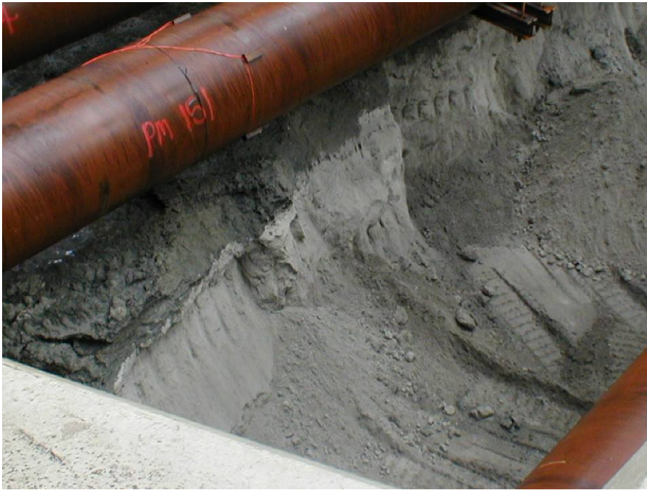
Figure 7.1 Sharp contact between the Upnor Formation (darker, above) and Thanet Formation (lighter, below), showing irregular topography of the boundary. From the Channel Tunnel Rail Link, Stratford box excavation after dewatering. (Copyright Jackie Skipper).
