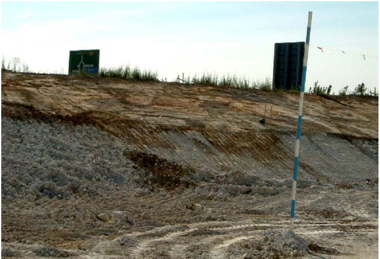
Figure 7.16. Excavation for the M4/A34 interchange at Chieveley, Berkshire revealing sand-filled channels in the Woolwich Formation, Laminated Beds (upper part of the view), and infilling karstic features in the underlying Chalk. (Copyright Jackie Skipper).
