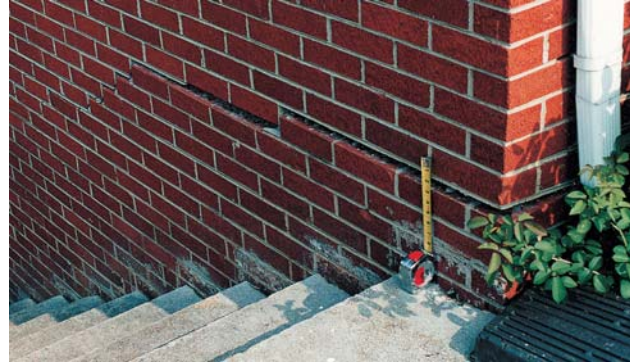
FIGURE 4 Damage to a home in East Tennessee caused by a cover-subsidence sinkhole. This damage developed slowly over several years. However, the area is underlain by limestone and has other characteristics of karst topography. Drilling showed a depression in the limestone surface in the area of the damage, and a slight depression in the ground surface could also be seen. (Photograph by Arthur J. Pettit, P.E. LaMoreaux & Associates, Inc. Used with permission.)
