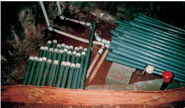
FIGURE 3 A monitoring network should always be installed in a show cave in order to avoid making significant changes in the cave environment. In the case of Kartchner Caverns in Arizona, such monitoring is particularly important because the relative humidity within the cave is close to 100% while outside the climate is very dry. During construction of the pathway, many pipes were laid down and covered by concrete. These pipes contain circuits that connect monitoring sensors within the cave with a computer in the main building. (Photograph courtesy of Arrigo A. Cigna.)
