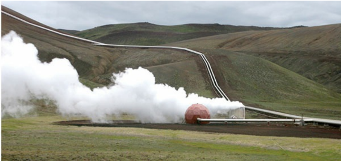
Figure 16.12 Geothermal well head (red geodesic dome) with steam rising from the adjoining relief valve and pipes feeding the superheated steam into the power-generating plant at the Krafla Volcano, Iceland.
