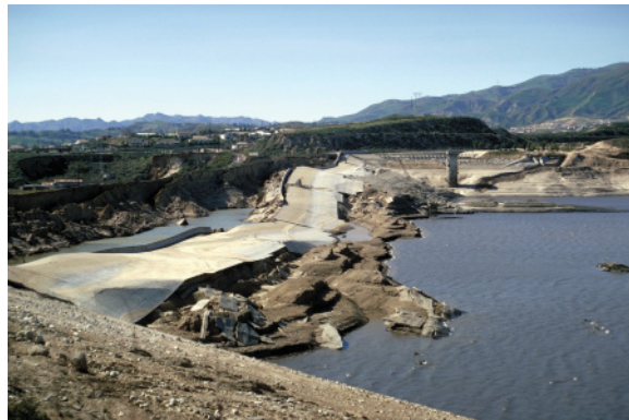
Plate B12.3a Damage to the Van Norman (Lower San Fernando) Dam, 1971. (From the Karl Steinbrugge Collection, courtesy of the National Information Service for Earthquake Engineering, EERC, University of California, Berkeley.)
