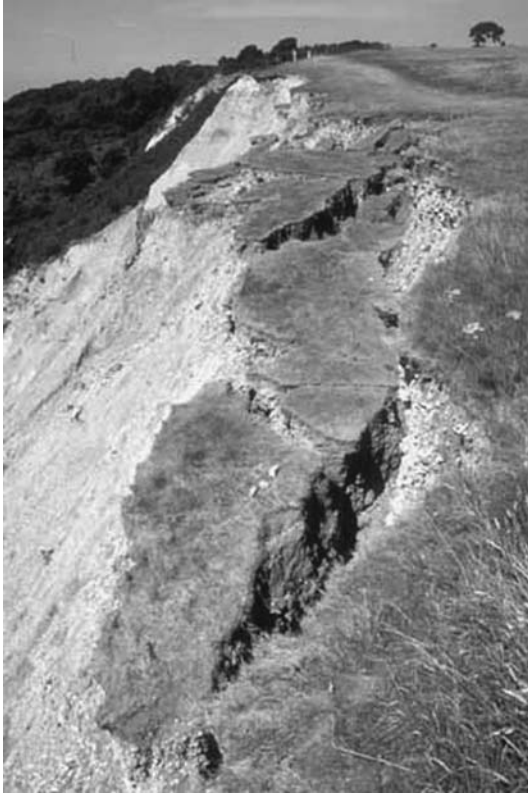
Figure 4.4 Breakaway on the cliff crest at Black Ven, near Lyme Regis in Dorset (cf. A in Figure 4.5)
