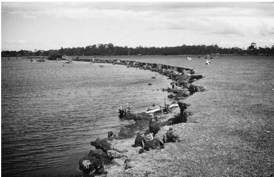
Figure 11.18 Shoreline erosion of previously formed swamp land on the shores of the Mitchell River silt jetties, Gippsland Lakes (see Figure 11.13)
