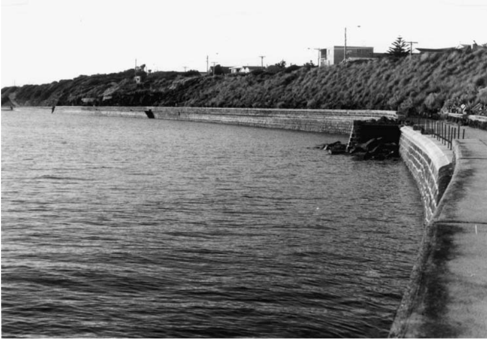
Figure 7.6 A sea wall and stabilised bluff at Black Rock in Port Phillip Bay, Australia, where the beach has disappeared as the result of reflection scour (as in Figure 7.5)
