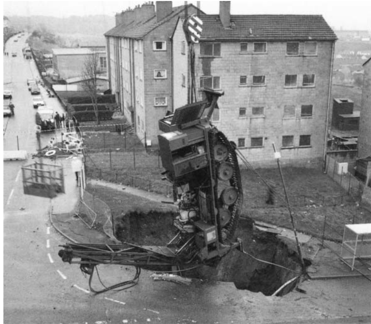
Figure 12.11 Collapse of capping material over an old concealed shaft in a modern urban area, UK. Source: Photograph by courtesy of IPR/25-36c British Geological Survey. © NERC. All rights reserved.
