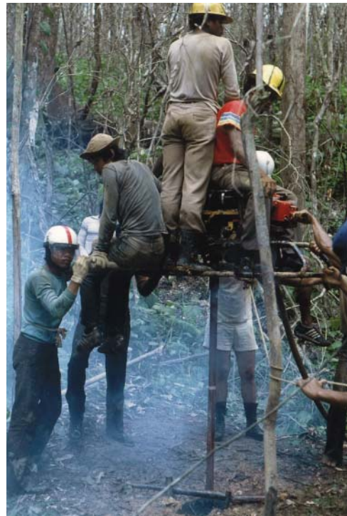
Figure 6.19 Portable drilling rig using manpower to exert downward pressure on the drill bit. In use in East Kalimantan, Indonesia. Source: Photograph by LPT.
