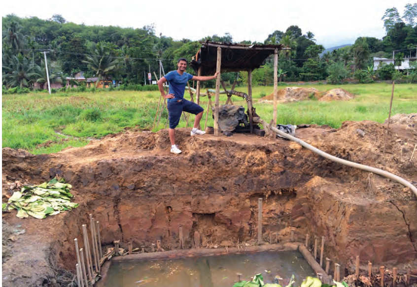
Group member, Shreyas V. Cotha, executive director of Bangalore-based C. Krishniah Chetty & Sons, stands at the top of a shallow pit in the Ratnapura area. Water seepage is a constant problem and must be pumped or bailed out. (Photo: Cynthia Unninayar)
