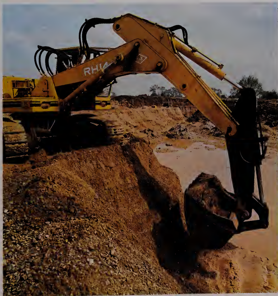
Below: Mechanical excavator quarrying ragstone, a sedimentary rock used in the building industry
