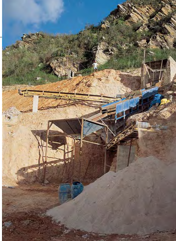
Figure 18. Fragments of gem-quality Paraíba tourmaline are occasionally recovered from stockpiled tailings, as well as from alluvial and colluvial material, at the São José da Batalha mine. This newly constructed processing plant will separate gravel-sized material from colluvium; the gravel will undergo further concentration at another nearby plant. Photo by Brendan Laurs.
