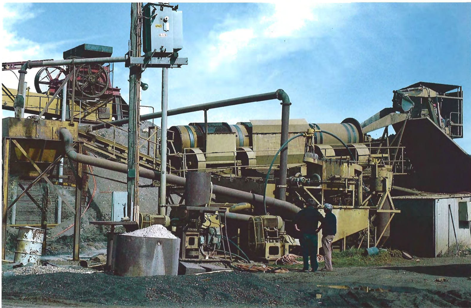
Figure 5. A mechanized processing and recovery plant at Kings Plan, Inverell, in the New England fields.
