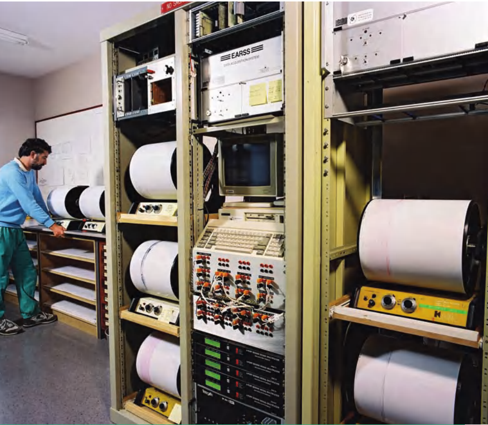
Seismic recording equipment, part of the Earthquake Arrival Recording Seismic System (EARSS) in New Zealand ( New Zealand © GNS Science/SSPL/ The Image )
