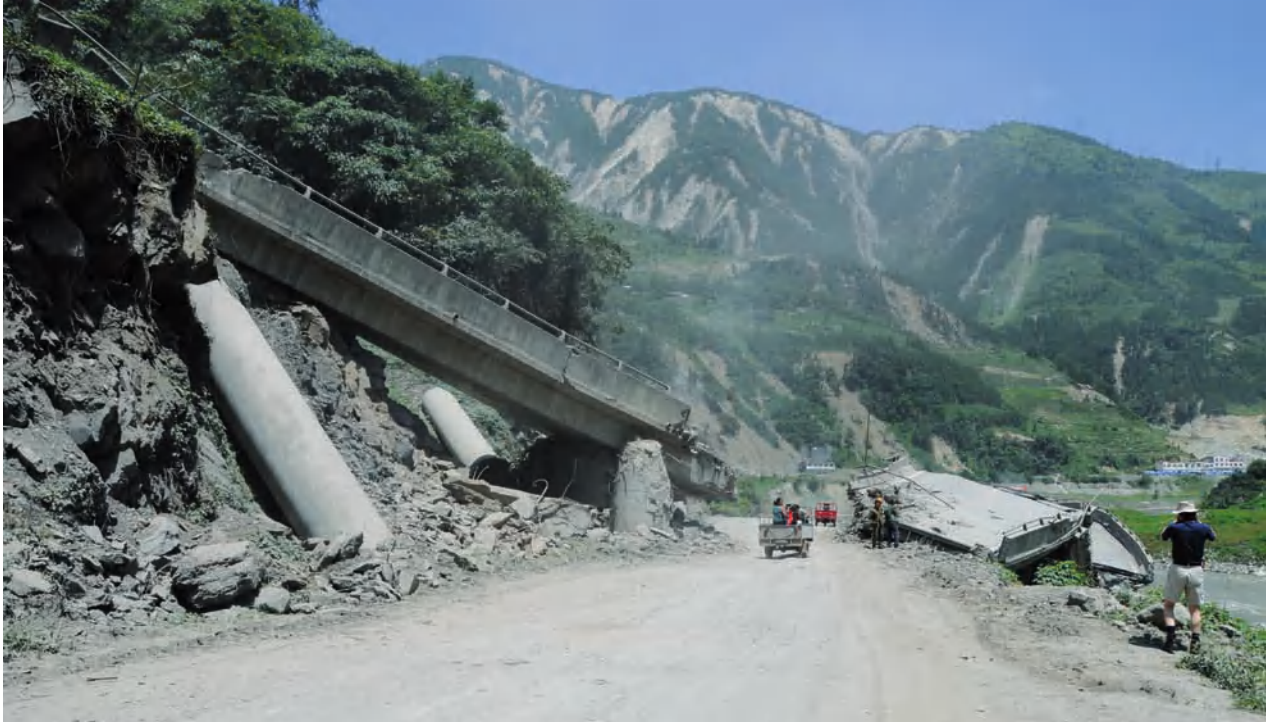
Damage from ground shaking and landslides in Yingxiu, Sichuan Province, China, from May 12, 2008, magnitude 7.9 earthquake (T. Kusky)
