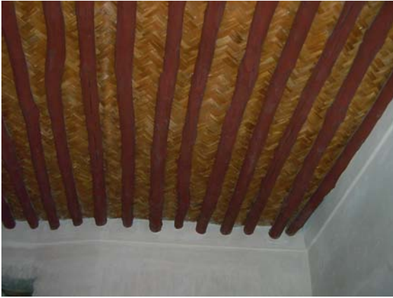
Building Construction. Fig. 7 Roof structure (Dubai) beams, mats, and mud as topping (photo by the author).
