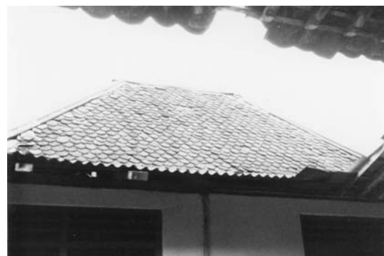
Architecture in Java. Fig. 4 Photo image of a limasan roof (author’s collection).
