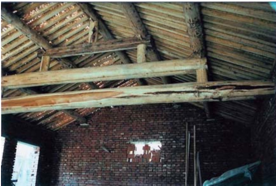
Building Construction. Fig. 8 Support of a roof in China (photo by the author).
