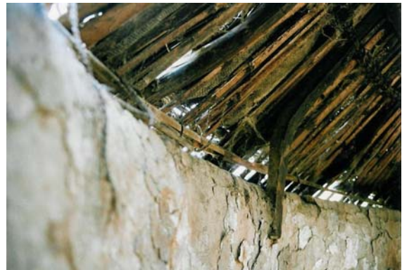
Building Construction. Fig. 21 Detail: corner element in a Bungha roof (photo by the author).
