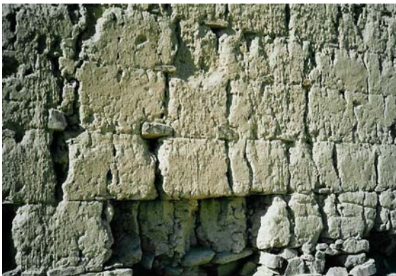
Building Construction. Fig. 5 Detail of the rammed earth blocks (photo by the author).
