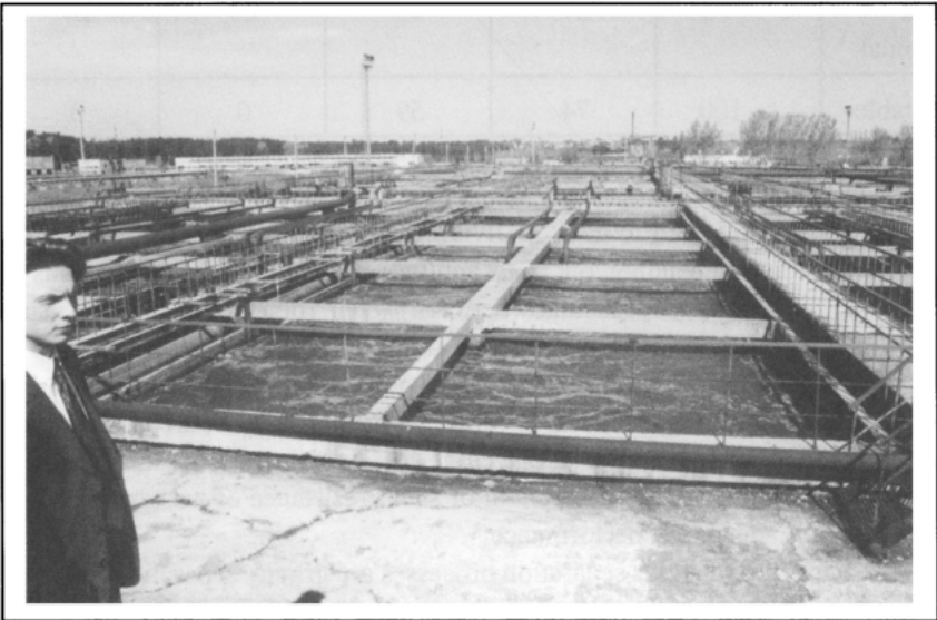
Figure 45. Rectangular settling basins in operation.
