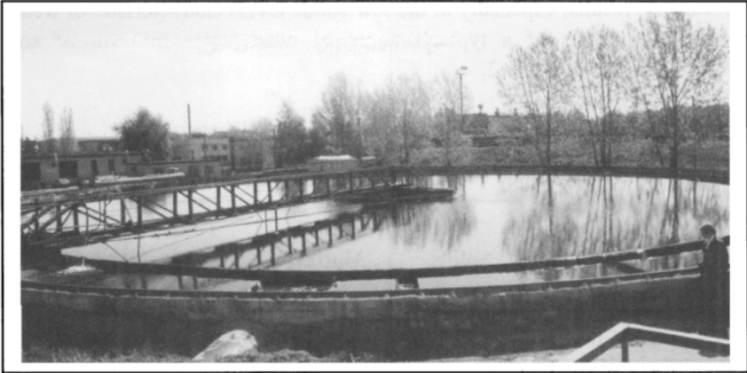
Figure 44. Clarifier in operation in a wastewater treatment plant at the Avtovaz auto-making plant in Russia.
