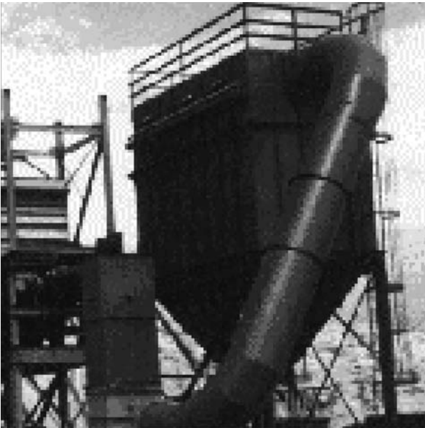
Figure 1-6. Baghouse dust collector
