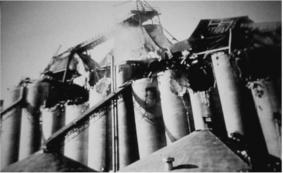
Figure 1-2. Silos destroyed in grain elevator explosion.
