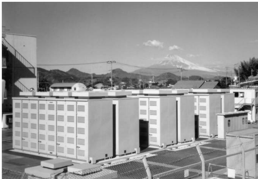
FIGURE 40.16 A photograph a 6 MW/ 48 MWh NGK sodium/sulfur battery system that is operating in a load-leveling mode at Ohito, Japan. This battery is one of the two largest sodium/sulfur batteries ever built and has been operating since early 1998 ( Courtesy of Tokyo Electric Power Company and NGK Insulators, Ltd. ).
