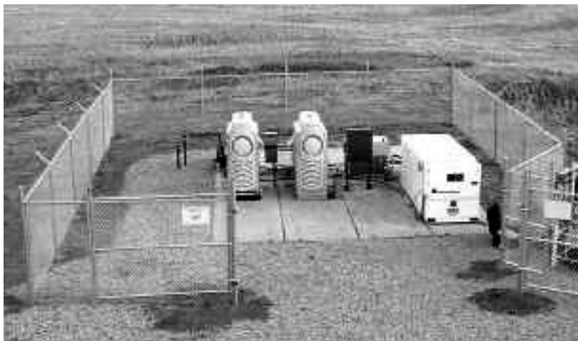
FIGURE 39.15 Aerial view of the PowerBlock® module with two microturbines near the Denver International Airport. (Source: From Reference 22.)
