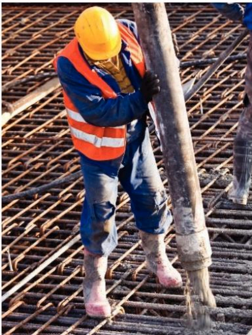
▲ The builder pours concrete into the gaps between the steel rods. The concrete sets hard.
