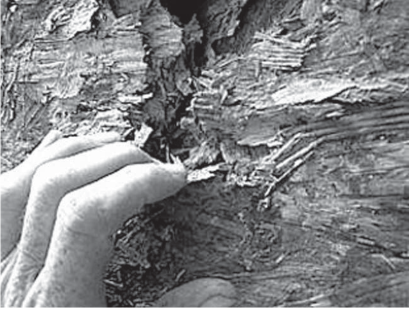
Wall sheathing on a six-year-old house that was clad with exterior insulating finishing system, showing serious rot.
