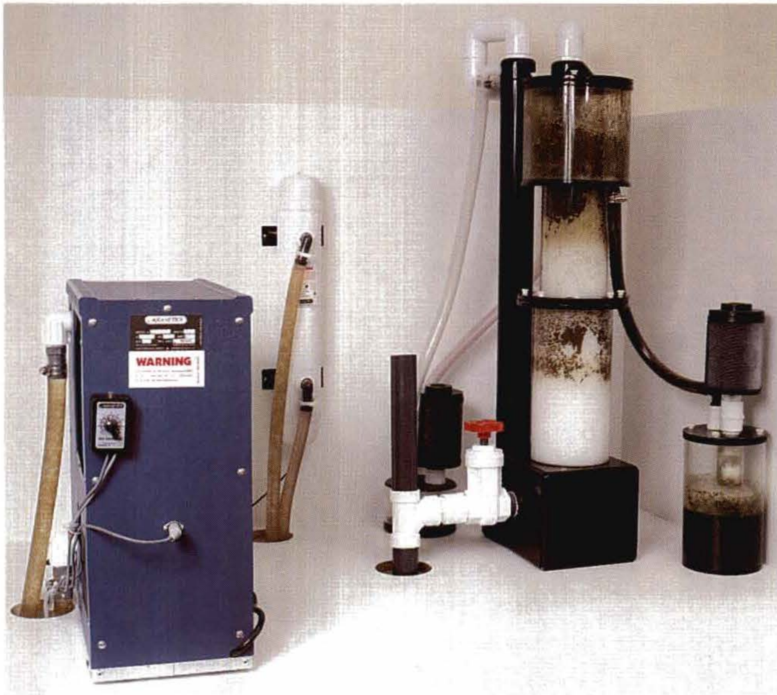
The behind-the-tank utility room has a large downdraft skimmer, UV sterilizer and heavy-duty chiller, all fed from a 90-gallon sump via a 150-gallon live-sand refugium.
