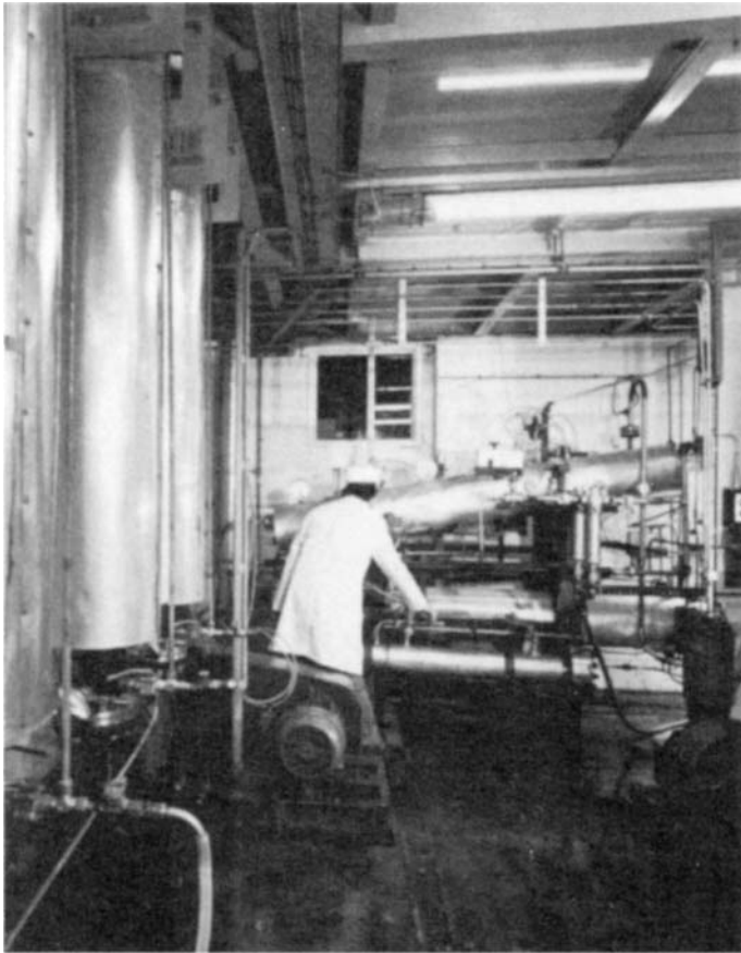
Figure 2-6 CO 2 extraction plant.
