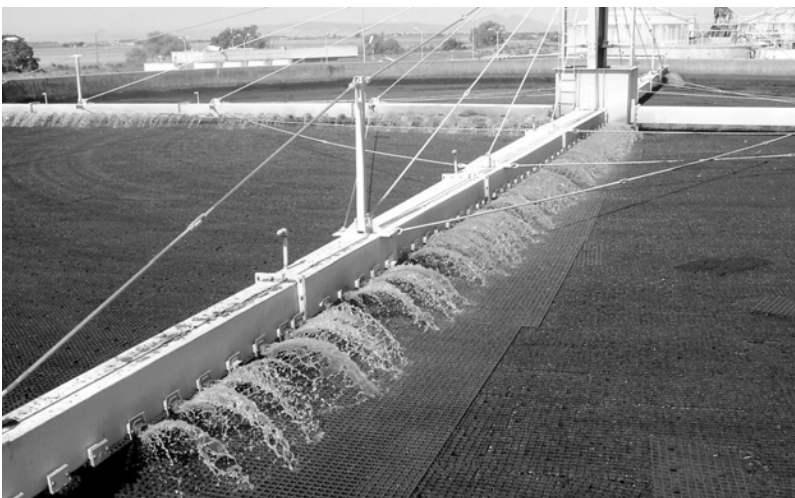
Figure 7.5 Trickling filter distribution system and plastic media.
