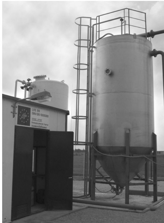
Figure 7.12 Tertiary moving bed sand filter (DynaSand) filter installed before ozonation of recycled water: demonstration plant for agricultural irrigation and aquifer recharge near Thessaloniki, Greece.
