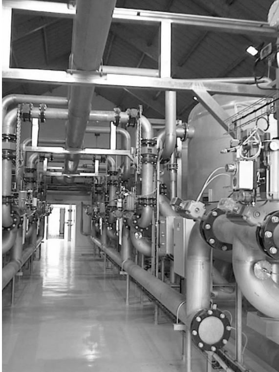
Figure 7.11 Pressurized tertiary sand filter (Courtesy of Degrémont).
