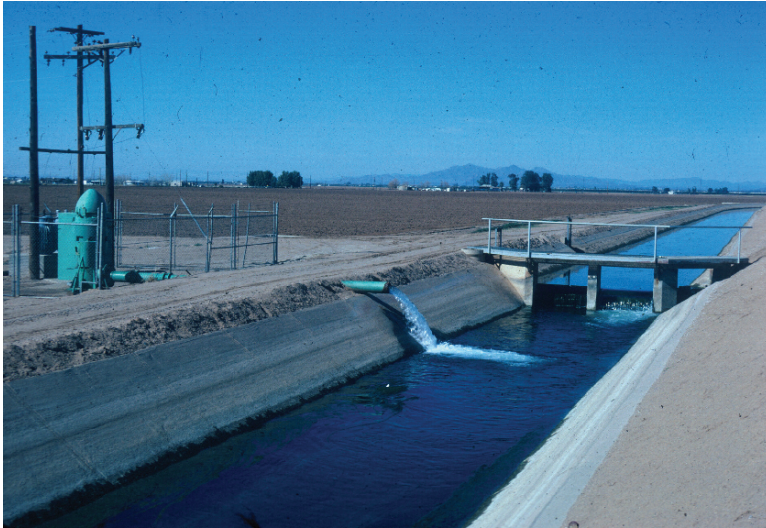
Fig. 5.10 Pumping groundwater into the (downstream) part of the conveyance systems improves the operational flexibility and control of the groundwater table
