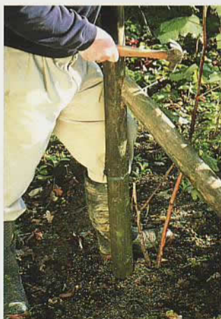
2 Fix another strainer post at a 45-degree angle in order to support the upright. Place this on the side the wire is to run and nail it firmly.
