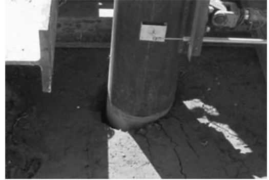
Figure 18. Photograph of a gap formation behind the pile (the pile is deflected laterally to the right and the gap is formed on the left of the pile in the photo).
