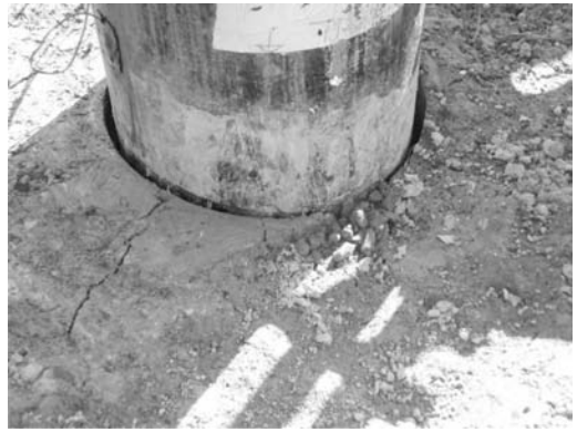
Figure 8. Gap opening after 8-mass loading.
