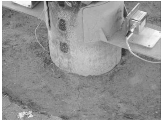
Figure 9. Gap disappeared after three weeks of rest and rain.
