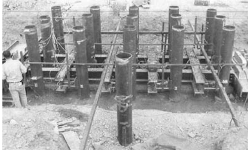
Figure 15. Full-scale lateral load test layout; a reference single pile in front of 3 \times 5 group pile.
