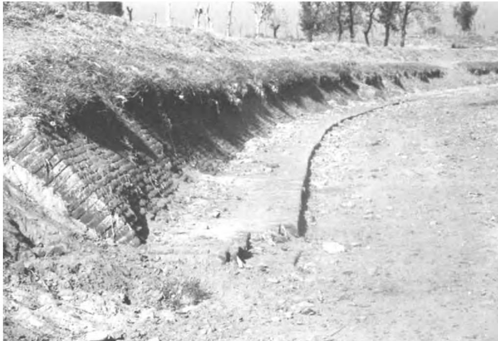
figure 6.10 Brick side lining stabilises the outside of a bend on the Maira Branch Canal in Pakistan
