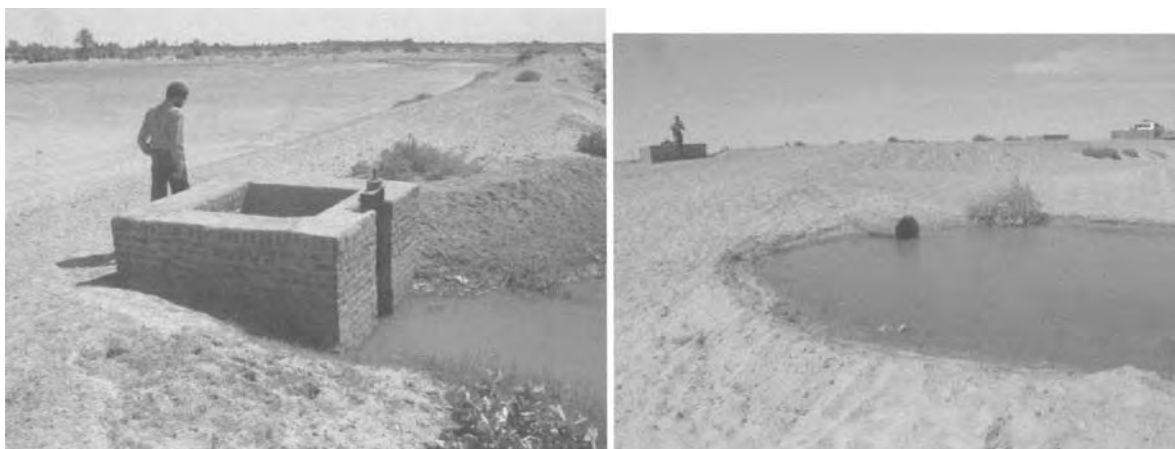
figure 7.4 A drop inlet turnout in Sudan – inlet gate and outlet pipe. Note the natural ‘onion’ shape of the outlet pool
