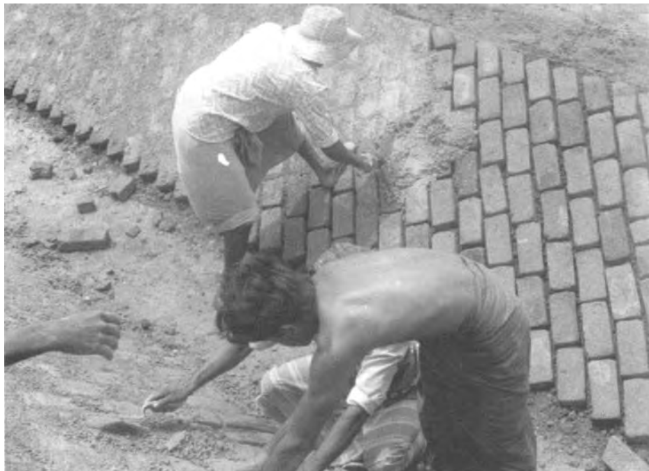
figure 9.4 Brick lining, Sri Lanka. Every joint is a potential source of leakage, but at least it's cheap
