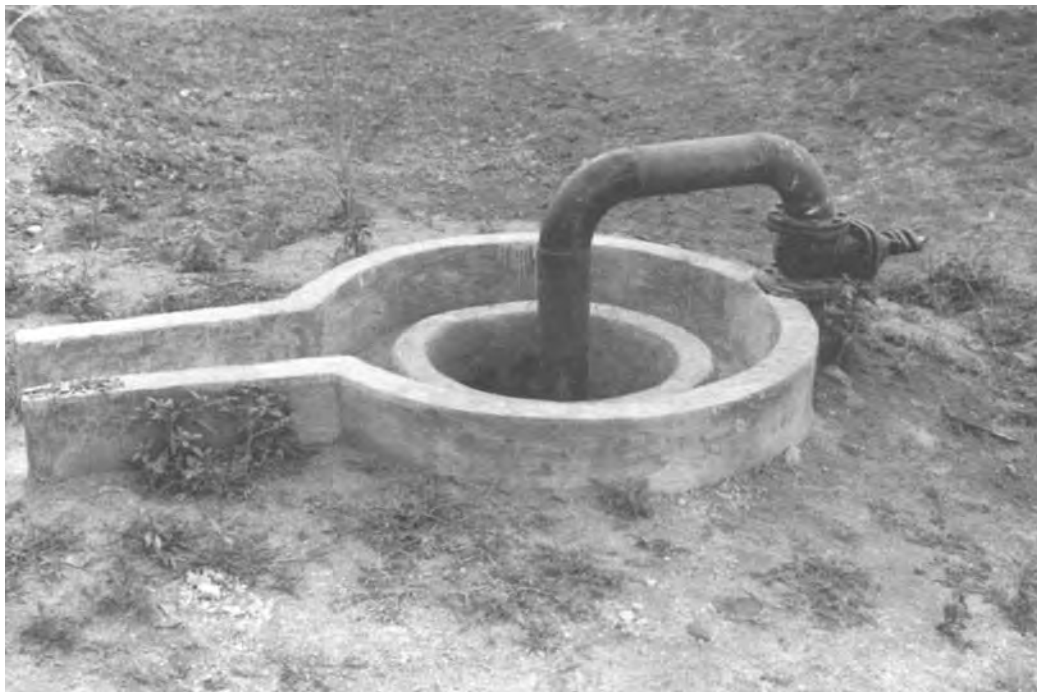
figure 8.13 A Beaumont circular weir outlet from a buried pipeline, Sulawesi
