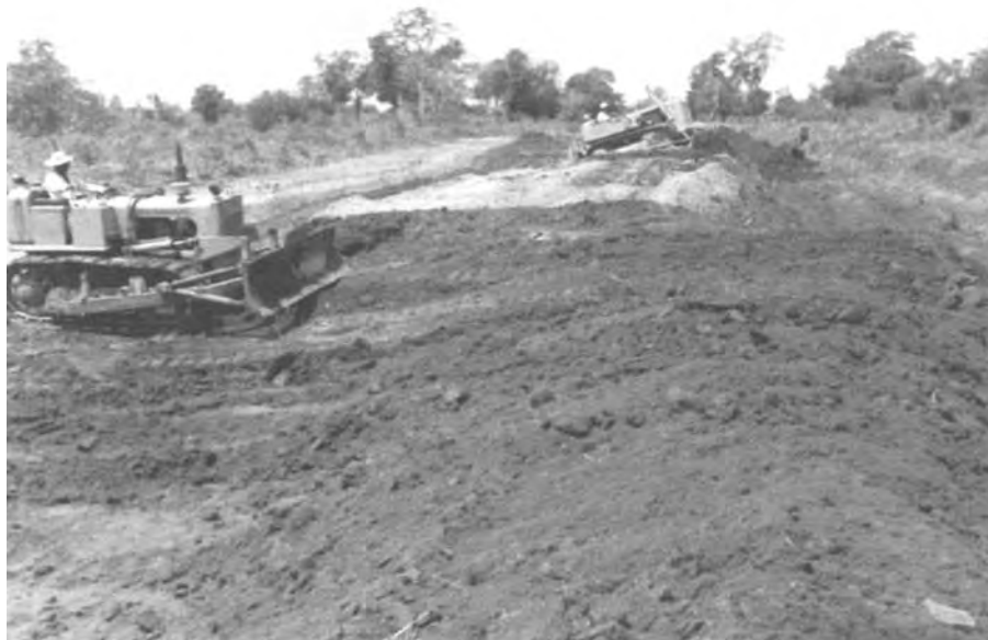
figure 9.14 How not to build a canal. Dozing up the banks without compaction, Sri Lanka
