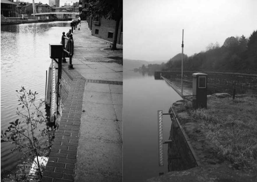
Fig. 2.7 Examples of pressure transducer installations with associated gauge boards (a) river level gauge (b) reservoir gauge (Sene 2008)
