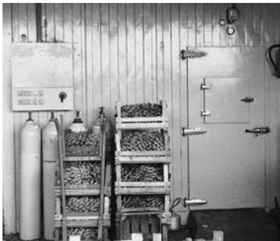
Figure 10.4 Small local banana ripening room in Brazil showing large ethylene cylinders connected to an injection system.
