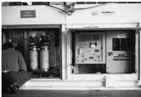
Figure 7.13 Nitrogen generators in use at a commercial controlled atmosphere store in the UK.
