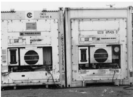
Figure 11.4 Packed controlled atmosphere reefer container plugged in to the mains electricity awaiting loading on the dockside in Castries, St Lucia, in 1998.
