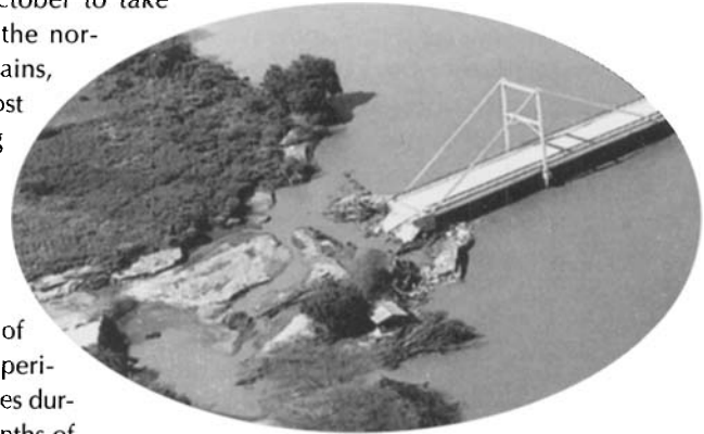
Washed out bridge on Kenya's main highway. (Photo courtesy of the United States Marine Corps/ U.S. Joint Task Force, Kenya)
