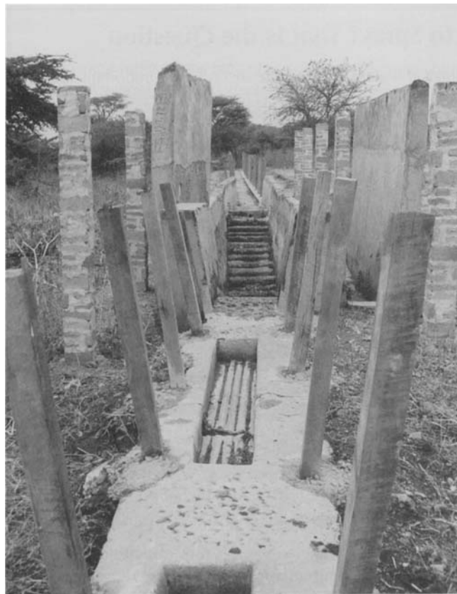
Figure 8-9. Many tick dipping stations have been abandoned in Africa. In this case, the dip was found to be unworkable because of poor construction design. Among other things, the walls of the dip were too far apart, allowing cattle to turn around in the dipping tank and impede the flow of oncoming cattle. (Photo by Dr. David M. Sherman)
