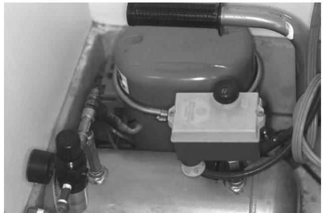
FIGURE 1.23. Remotely located stand-alone compressor.
