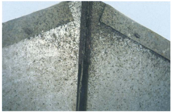
FIGURE 5.14 Fecal spots, indicative of cimicid activity, along seams of nesting boxes of laying hens in a poultry house heavily infested with Cimex lectularius . (Photo by G. R. Mullen)
